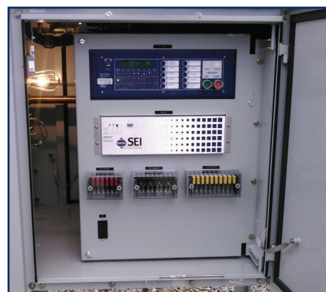
Control panel that directs the wiring contained within the substation.
